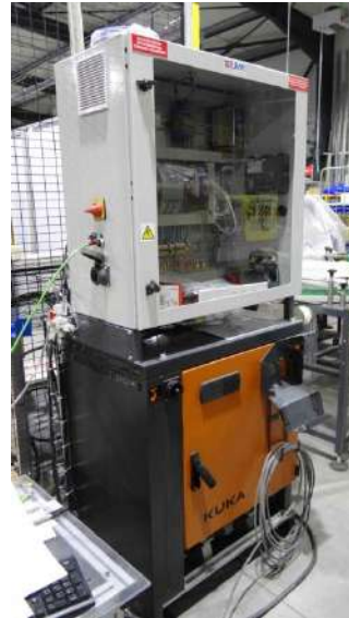
Power and control box & robot control cabinet
